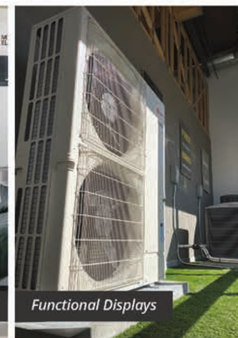
Ductless Mini-Split Installations
