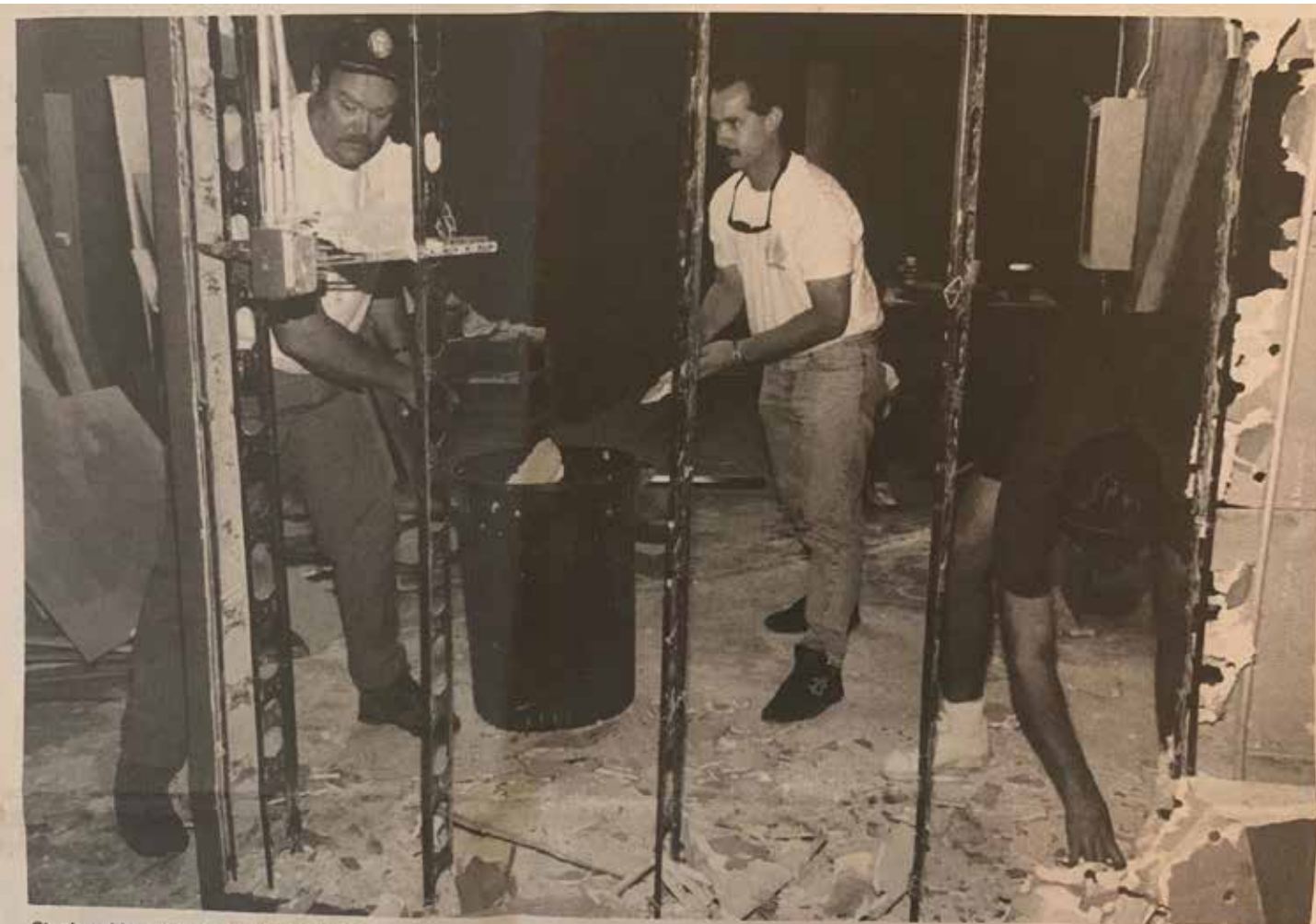
Stephen Munteer/Scottsdale Progress Rural/Metro fire chief Karl Keierleber (left) and firefighters Greg Marlar and Dan Bunce take down a wall recently as part of their work in preparing a 10,000-square-foot facility at Tower Plaza for construction of the Valley Youth Theatre's first permanent home. The firemen, who volunteered to help on the project, are just three examples of the community support given the Valley Youth Theatre in its attempts to open the theater by mid-August.
